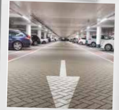
2013 Decentralised emergency lighting integrated into luminaires.
